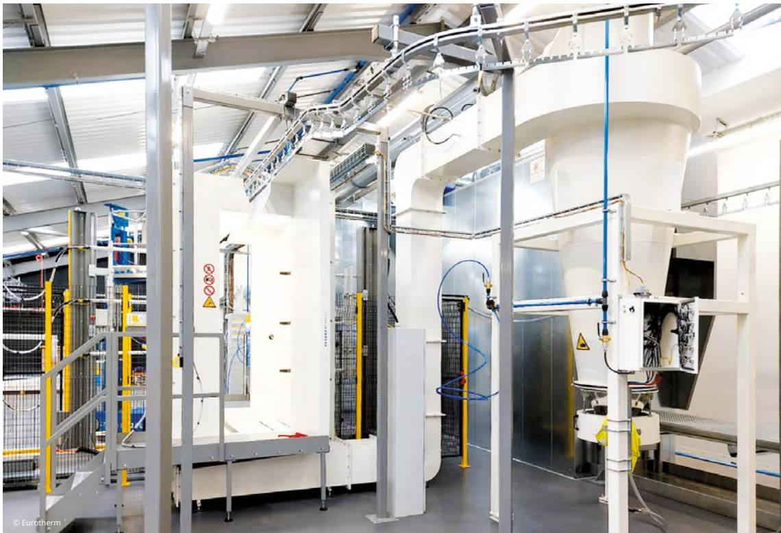
Overview of the powder coating booth supplied by Wagner.
