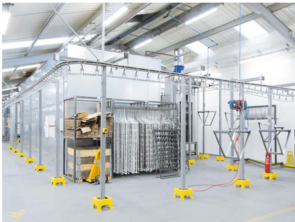
Overview of the powder coating line designed by Eurotherm (Turin, Italy) and installed by PFS Paint Finishing Systems.
